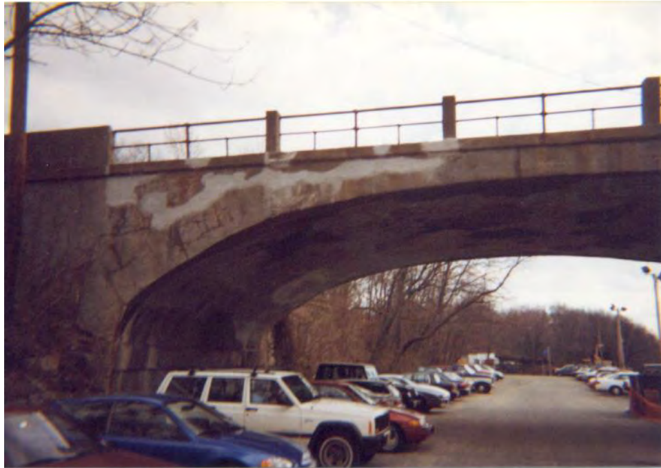
Photo 3-9: Looking south at the north face of the east span arch ring and spandrel wall. Note: Large areas of concrete repair work to the spandrel wall (light color in photo) under repair contract in 2000.
