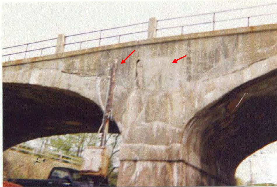
Photo 3-2: Looking south at north face of east and west arches at center pier. Note: Heavy medium cracking with efflorescence and leaching in arches, spandrel walls and piers and spalls in spandrel wall (arrows). Photo taken prior to repairs in 2000.
