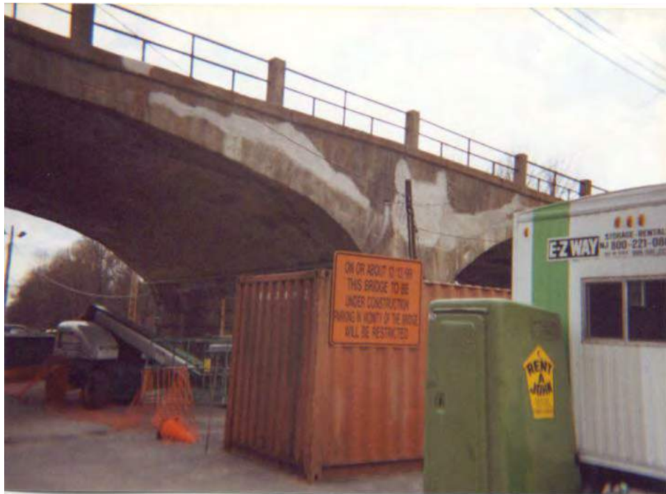
Photo 3-7: Looking southwest at spandrel at center pier for east and west spans. Note: Large concrete repair areas (light gray color in photo) done under repair contract in 2000.
