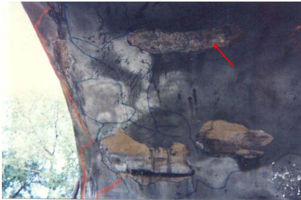
Photo 3-4: Looking east at north edge of east span arch ring underside. Note: Spalled gunite treatments and large spall in underside of arch ring (arrow). Photo taken prior to repairs in 2000.
