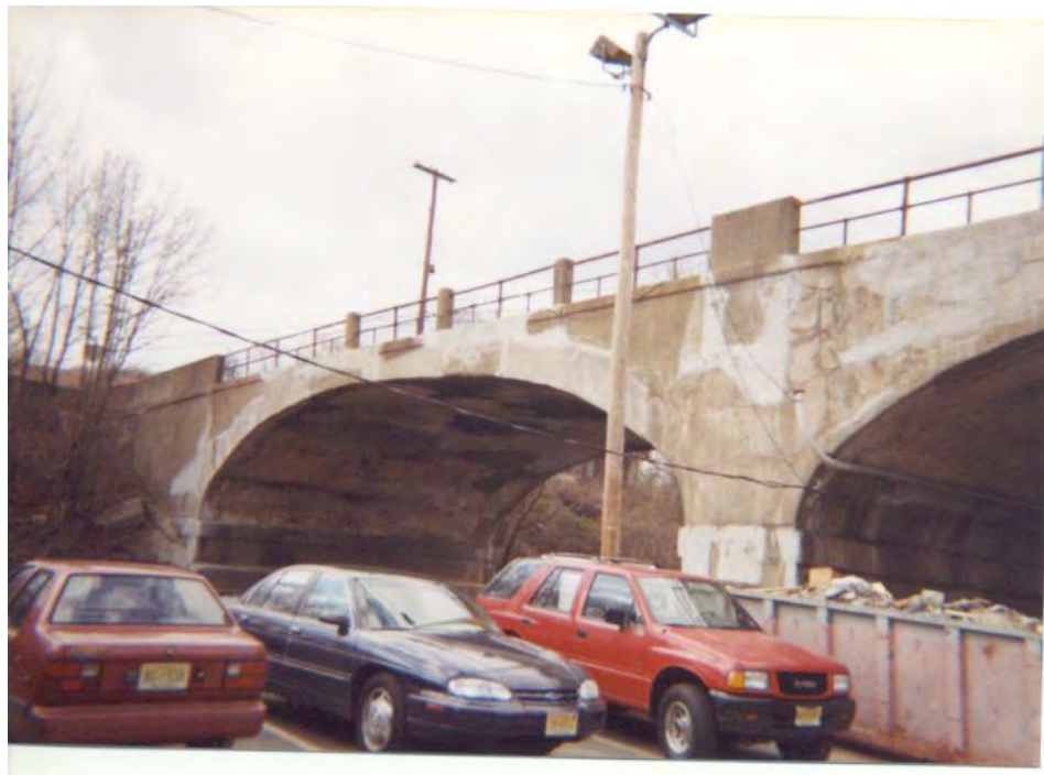
Photo 3-8: Looking northwest at the south face spandrel wall, center pier and the edge of the west span arch ring. Note: Large areas of concrete repair done under repair contract in 2000.
