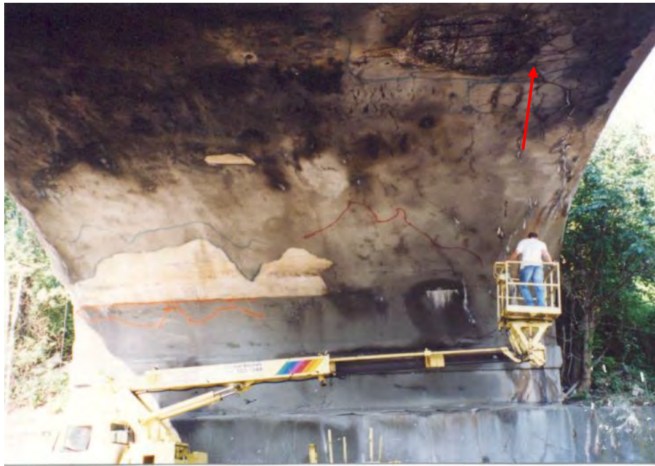
Photo 3-5: Looking west at large spall with exposed corroded reinforcing bars in north half of the west span arch ring underside (arrow). Photo taken prior to repairs in 2000.
