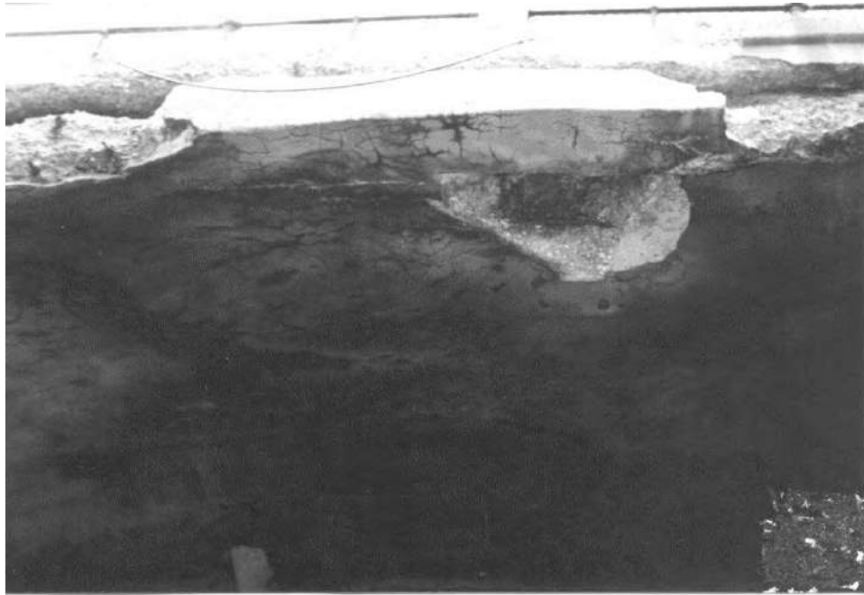
Photo 3-3: Looking northwest and up at the edge of the underside of the west span arch ring over NJ TRANSIT tracks. Note large spalls in underside and edge of arch ring. Photo taken prior to repairs in 2000.
