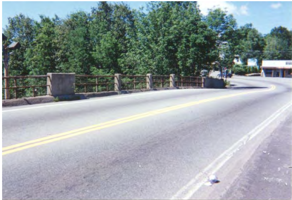
Photo 3-12: Looking southeast at the west span roadway over NJ TRANSIT Montclair-Boonton Line. Note: Bridge deck geometry has an inadequate to curb-to-curb width of 29 feet 7 inches (present design standards require 34-foot minimum).
