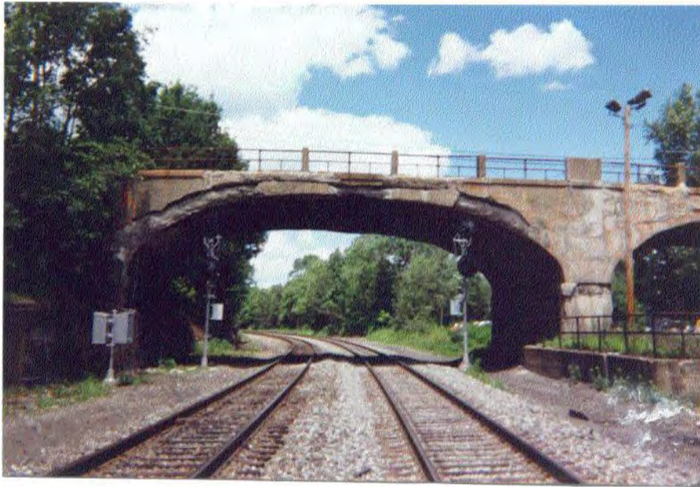
Photo 3-1: Looking north at south fascia of the west arch over the NJ TRANSIT Montclair-Boonton Line (formerly the DL&W Railroad). Note: Large area of the spandrel wall and edge of arch ring heavily spall (Photo taken prior to repairs in 2000).
