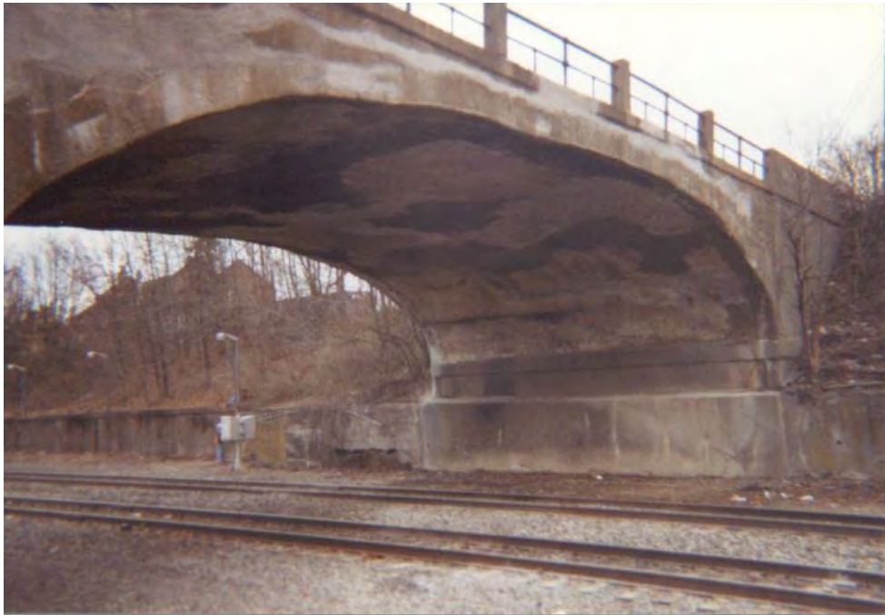
Photo 3-11: Looking southwest at the north face of the west span arch and spandrel wall. Note: Large area of concrete repairs to spandrel wall and arch ring under repair contract in 2000.
