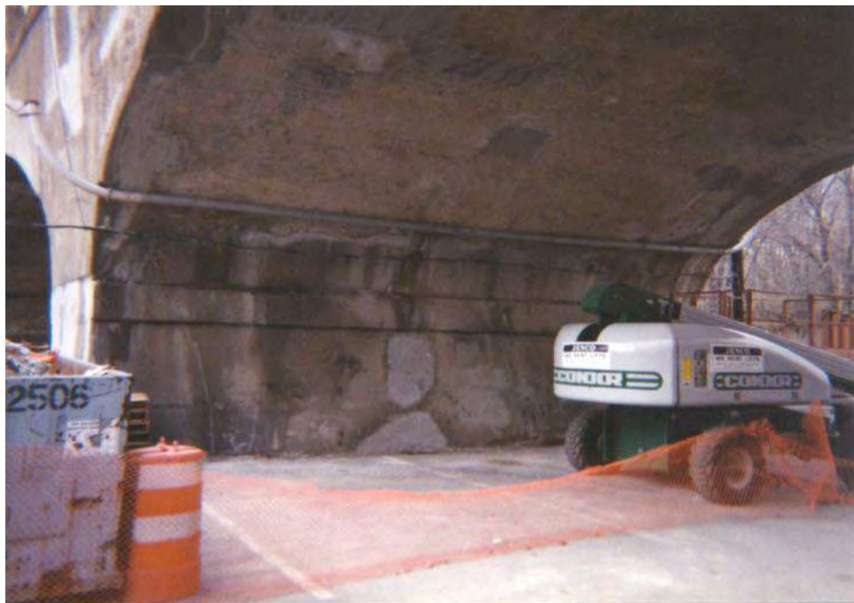
Photo 3-10: Looking northwest at the east face of the center pier. Note: Concrete repair work done under repair contract in 2000.
